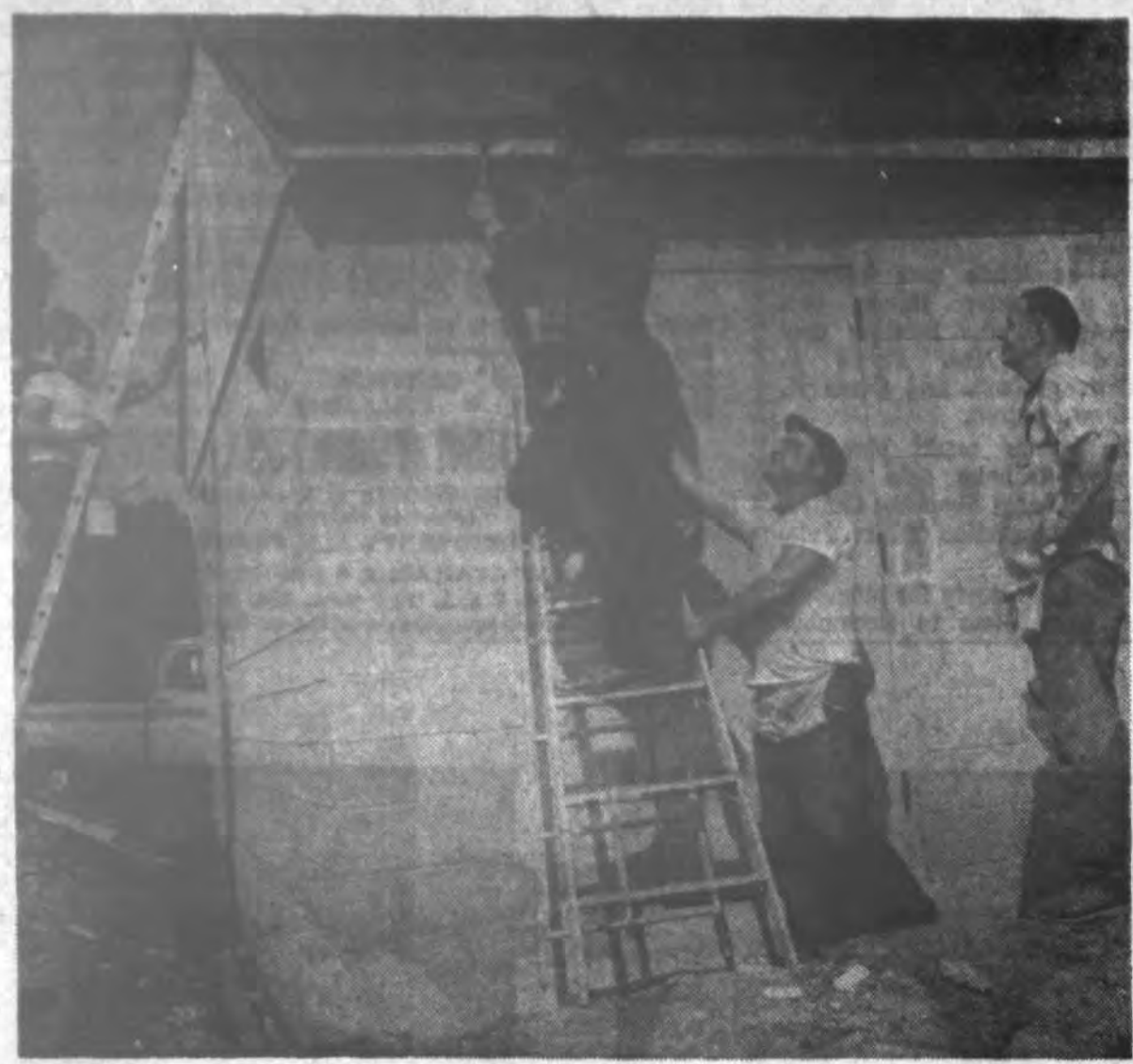
BUILDING NEARLY COMPLETED — Greenway-Verona Mills Fish and Game Club facility on Sholtz Road is nearly complete. Members are doing work themselves and hope to have project finished by November. Workers, from left, are: Carl Campbell, Greenway; Lawrence Dupre, Verona; Kenneth Millson, Verona Mills, and Frank Cieslewicz, Rome-Oneida Road. (Kate Peabody photo).
